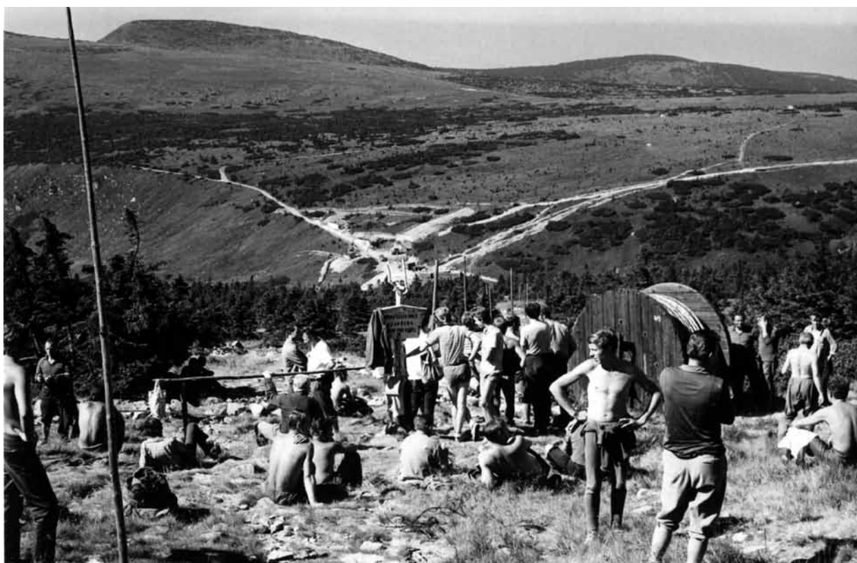
Laying cables from the Labská bouda Chalet to Martinova bouda and to the Sněžné jamy Cirques, probably in 1969. As with Mt. Sněžka the electric cable and water mains run from the Polish side, while the cable to the Sněžné jamy Cirques runs from the Czech side. Connecting Krkonoše to mains electricity and water has continued from 1965 until today. During these works the surface cabling has been replaced and nearly all of the previously unconnected localities have been electrified (of the large enclaves, the Klínové Boudy Chalets was connected in 2008). We must also mention the lines of telecommunication cables. Linear constructions are a sensitive matter, which are still carefully monitored (photo Miroslav Hladík)
