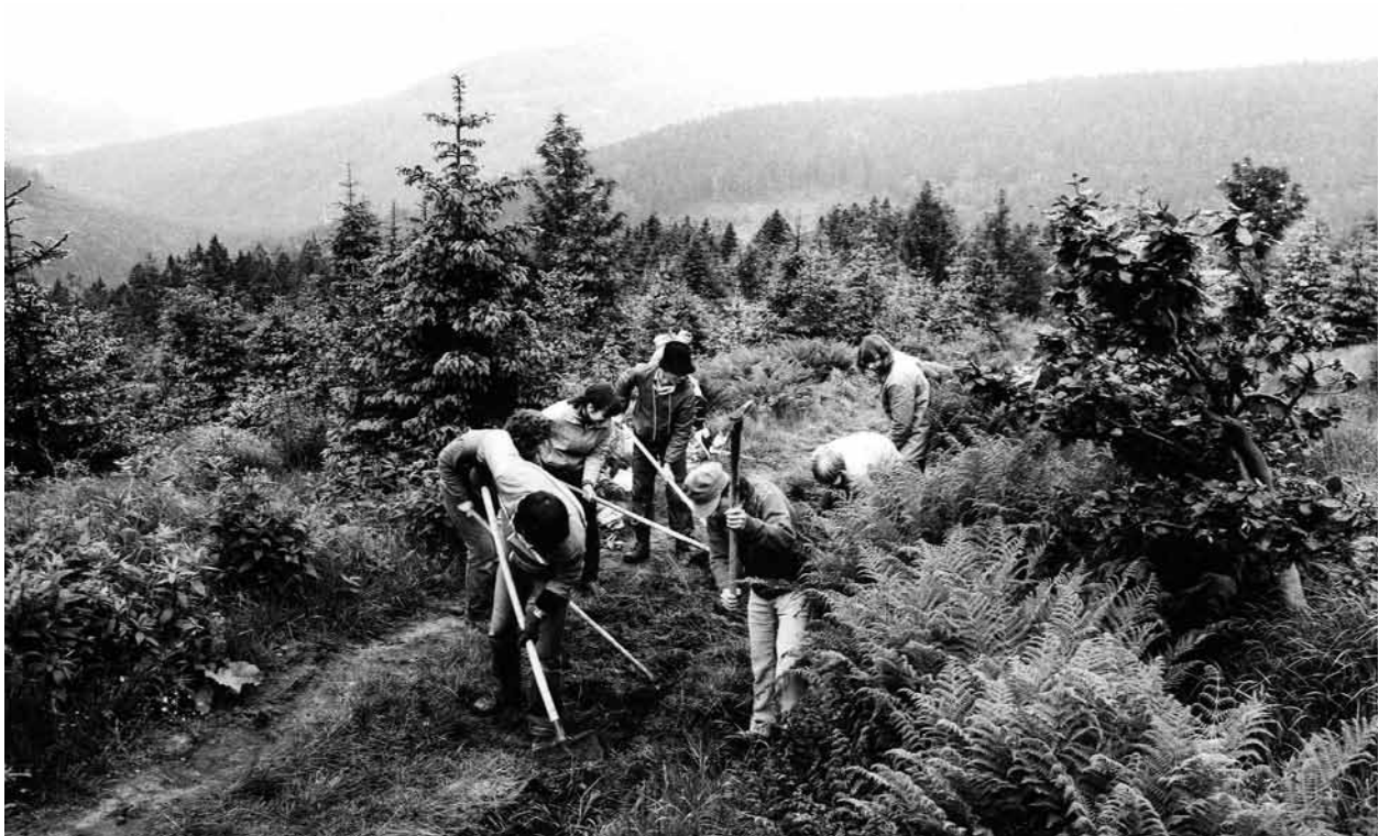
'Young Hands for Krkonoše' event – repairing the trail and its drainage between the Martinova and Labská bouda Chalets, 1984 (photo Jiří Bruník)
