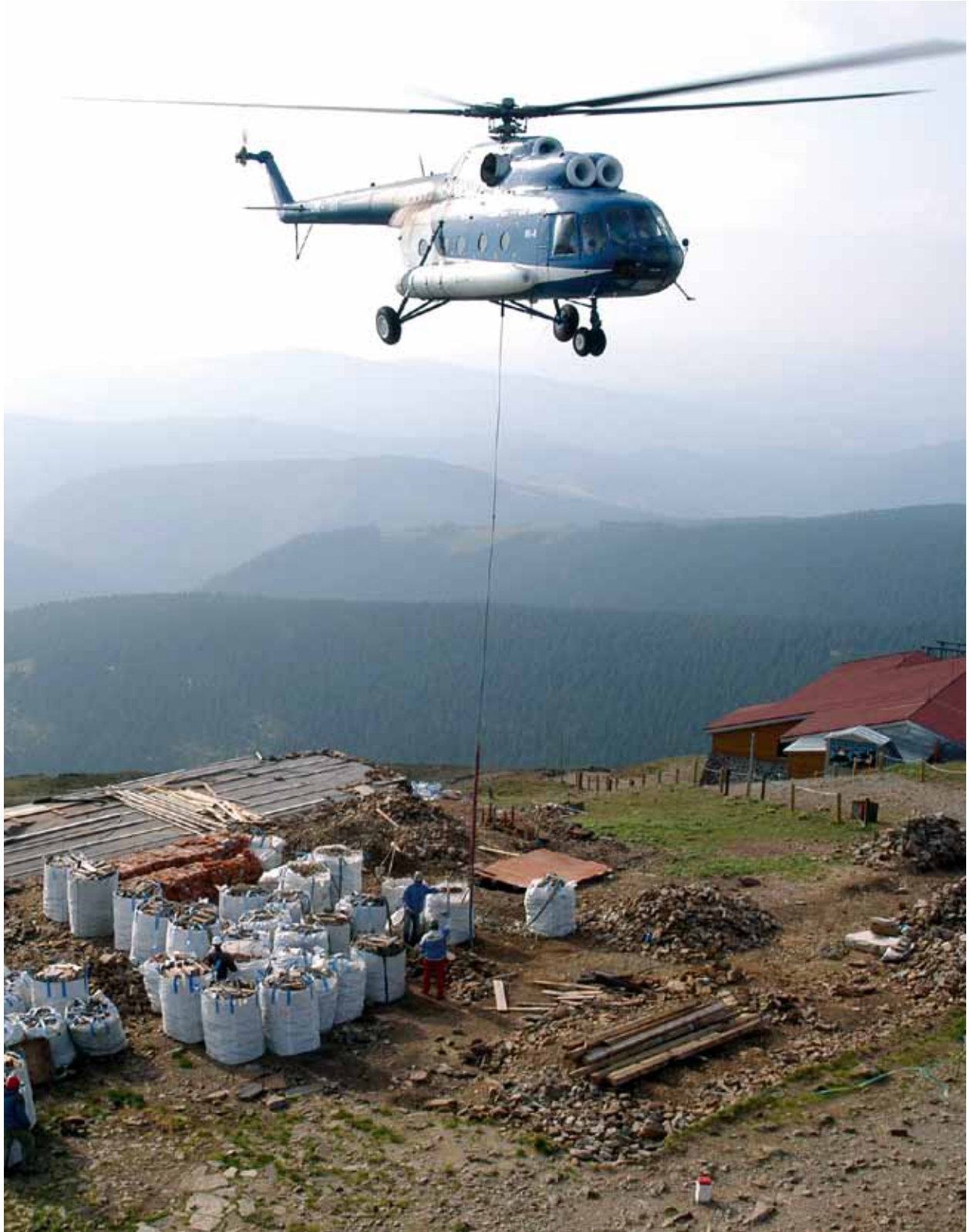
...and here it is dismantled and packed away. The helicopter was an invaluable helper during the demolition of the rundown Česká bouda Chalet and the following recultivation of the terrain by the workers of the Klimeš Construction Company. (photo Kamila Antošová)
