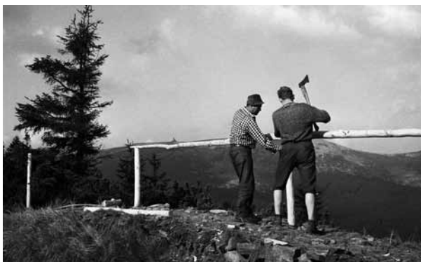
In addition to repairing the trails, effective measures were also taken to direct the movement of tourists. Here the Administration staff are building the Šmíd Vantage Point on the eastern slopes of Krkonoše. 1960s (photo Miroslav Hladík)
