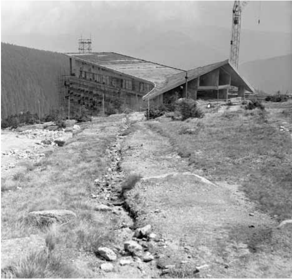
Damage to the terrain along the route of the water mains to the new Labská bouda Chalet (photo Jan Štursa)
