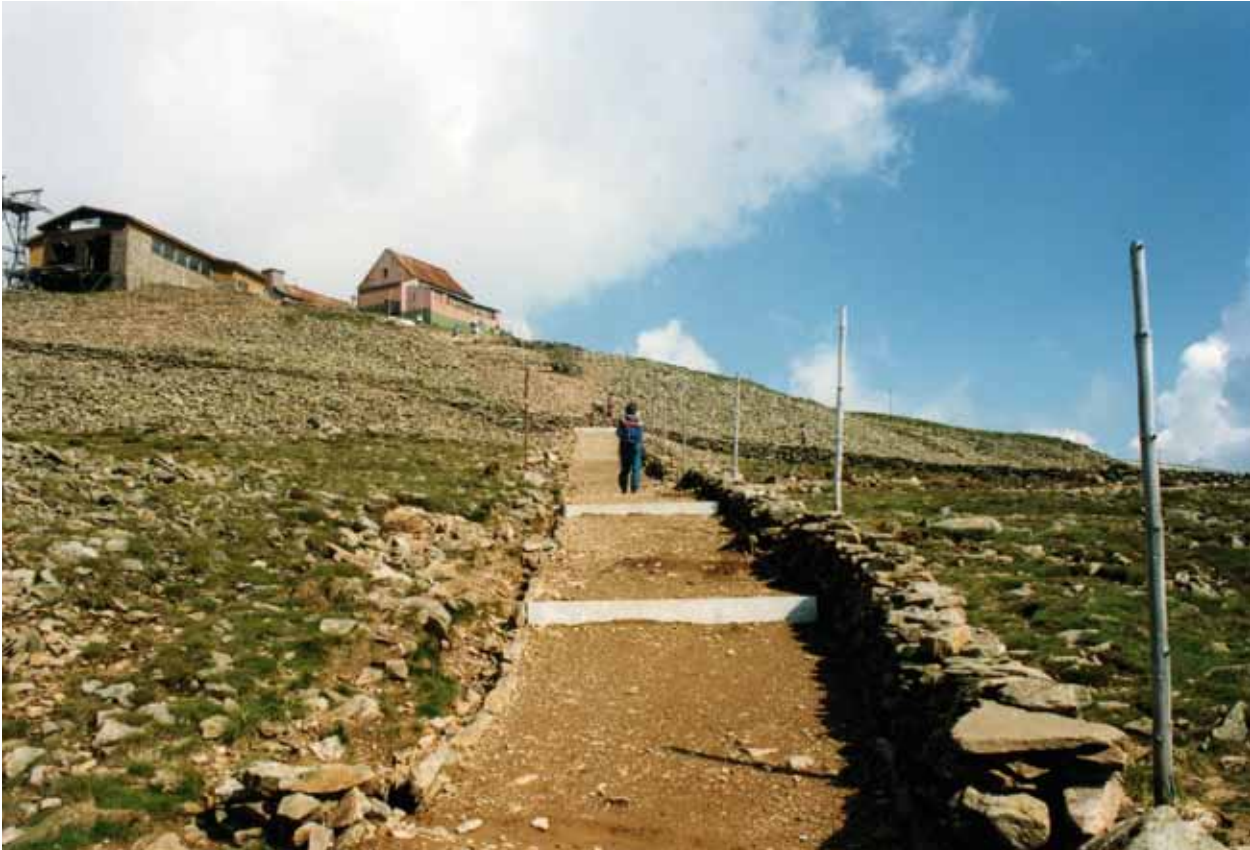
The overall appearance of the repaired trails is improved by the lateral stone walls, which are also effective in the fight to keep the tourists from straying away from the trail (this is the First Zone of the national park, with the strictest protection regime). The Česká bouda Chalet is still standing... (photo Jan Štursa)
