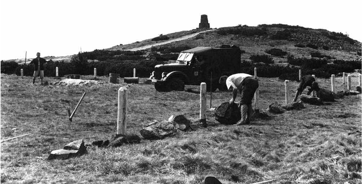
Building the car park at the Vrbatova bouda Chalet (photo Miroslav Hladík)
