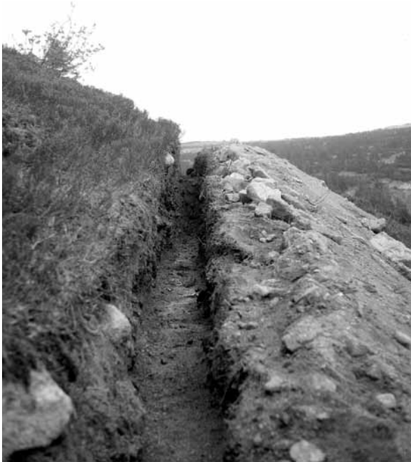
The badly-chosen route for the trench carrying waste from the biological septic tank at the new Labská bouda Chalet led directly into strictly protected Navorská jáma Cirque. The mistake was corrected in time and the trench was backfilled and restored to nature (photo Jan Štursa)
